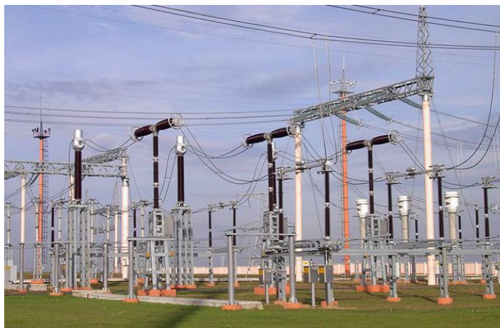
2. GL316 (SF 6 ) live tank circuit breaker in substation
